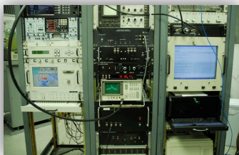
21 m Antenna Control System
