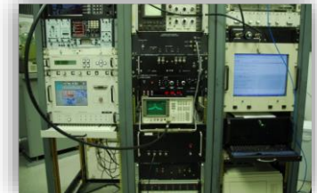
21 m Station Control System
